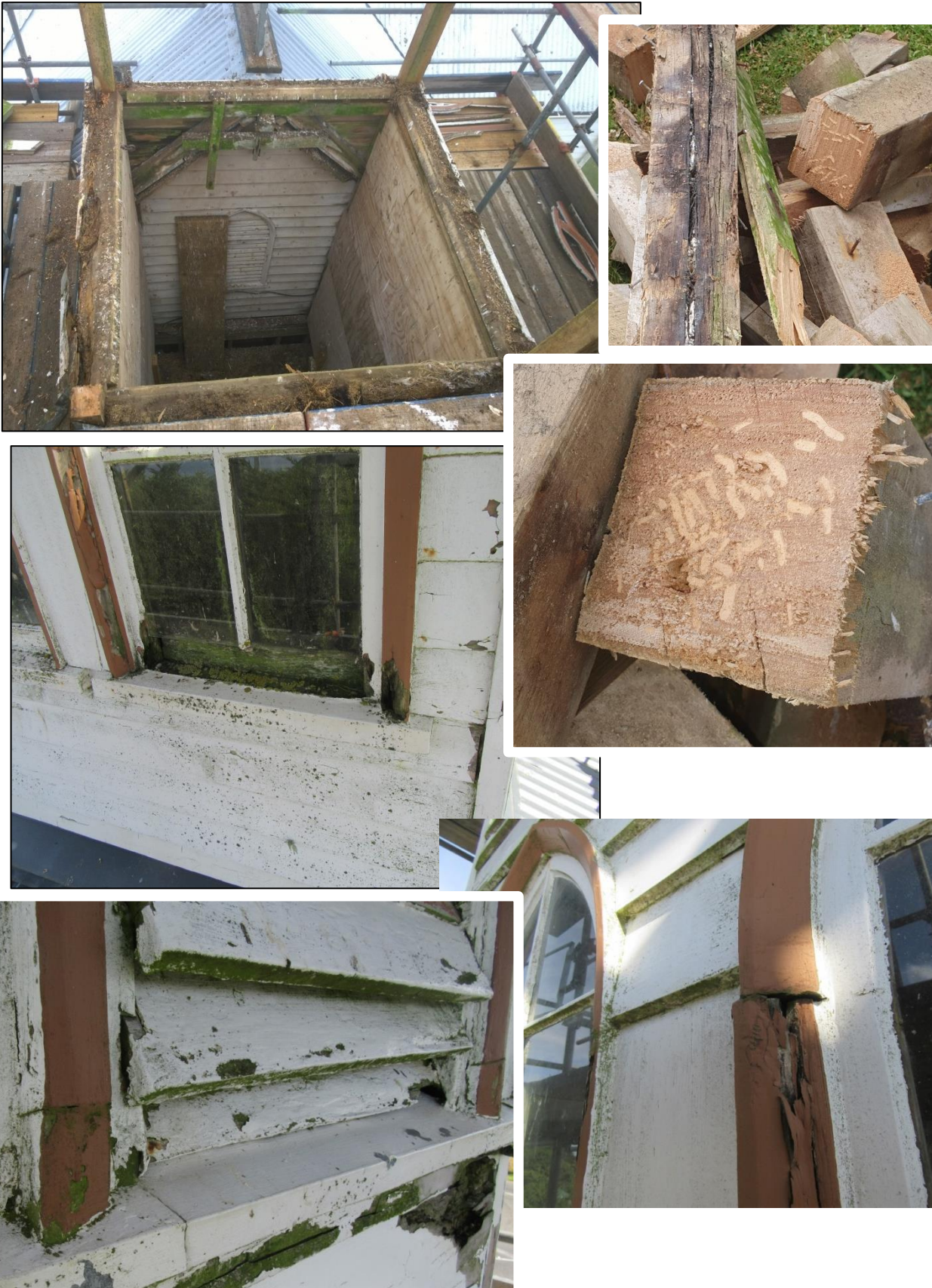
February 2020: The main support posts of the tower were badly riddled with borer and the windows and louvres badly decayed. The tower needed to be rebuilt.
